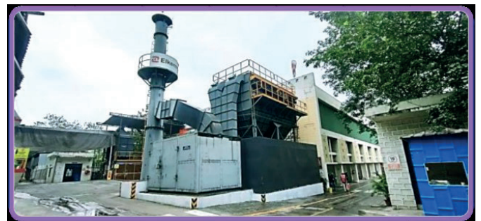
Photo-3: Dust Collection Silo with Barricades, Exhaust, Chimney and ID Fan Sound Enclosure
