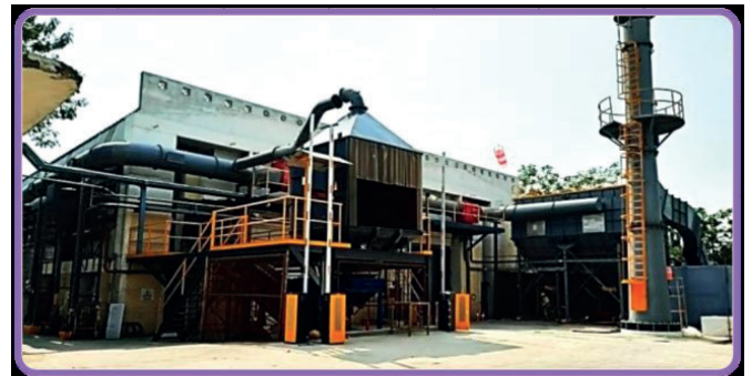
Photo-2: Fe-Si-Mg Slabs charging Hopper
