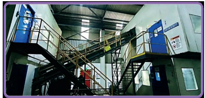
Photo-1: Vibrating Screen Acoustic Enclosure rooms & conveyors inside the Main Building
