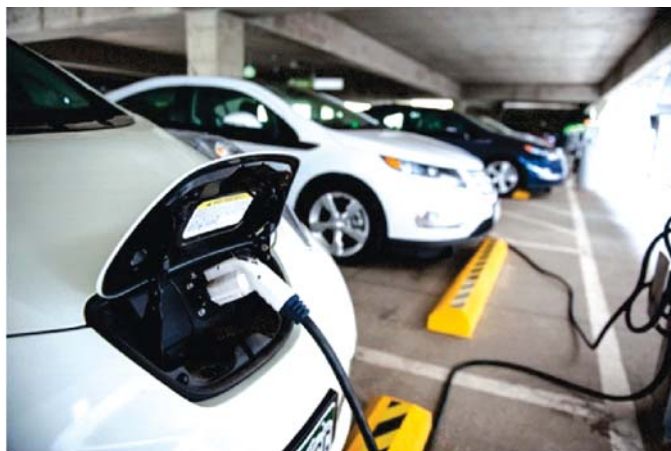
Electrical Vehicles (EV) charging station
