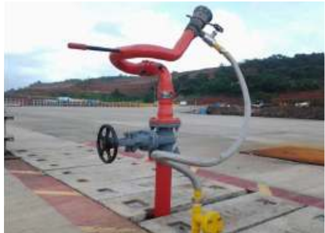
Fire Monitor on Cargo Jetty with Foam Concentrate Line
