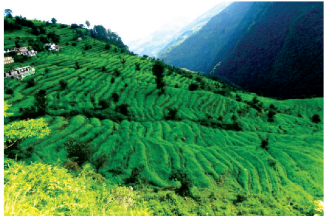
Slope stabilisation with provision of intermediate terraces in Lamgondi village, District Rudraprayag
