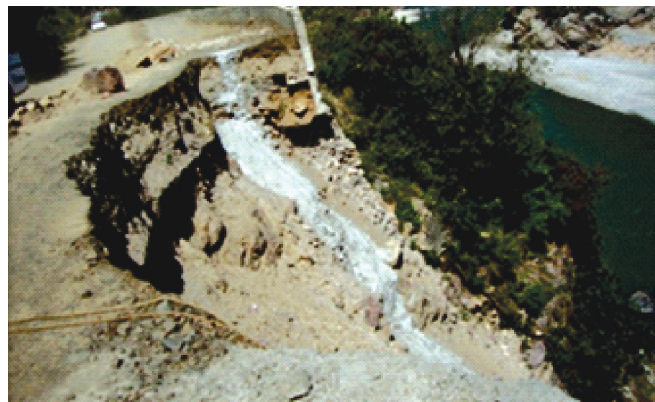
Landslide along a road due to an unstable slope, uncompacted fill and absence of a retaining structure.
