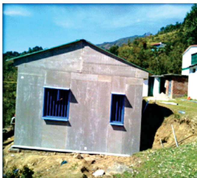
Aganwadi construction using prefabricated earthquake resistance structures at Bhiri village, District Rudraprayag
