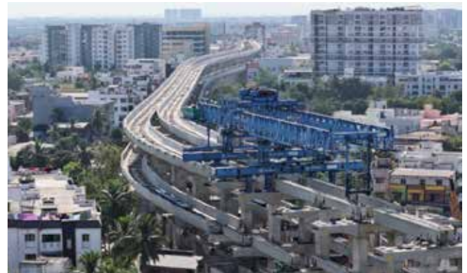
Double Decker section at PORUR
