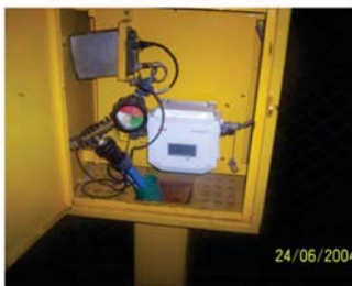
District Meter Cabin and display unit
