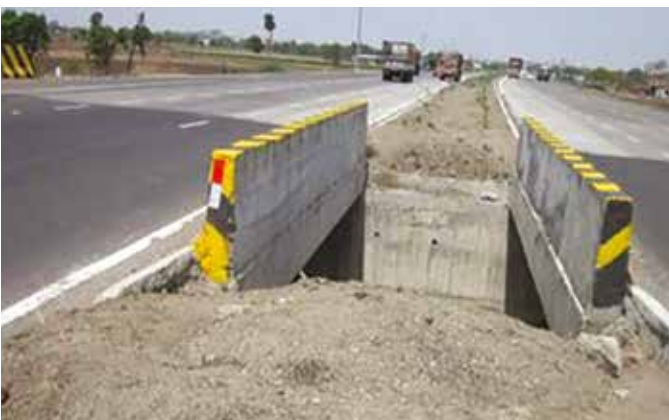
Un-protected minor bridge, vehicles can fall down between the parapets
