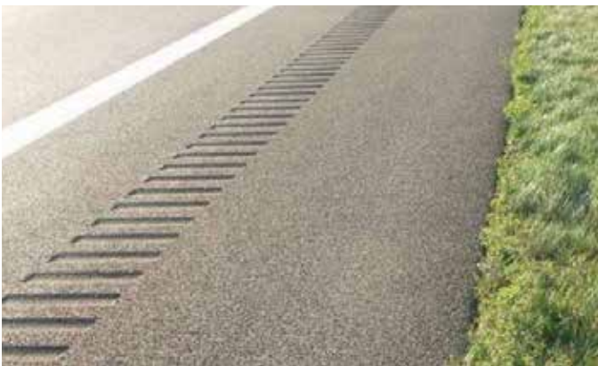
Rumble strips provided to alert driver of drifting away and carriageway and to prevent run-off crashes
