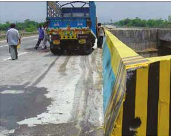
Abrupt placement of crash barriers especially concrete/ masonry with no crash cushion.
