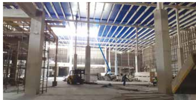
Photo-3, Snowpark and Family Entertainment Center Construction in progress (photo by rvgomeseria)
