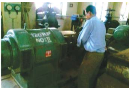
Energy Audit Work
