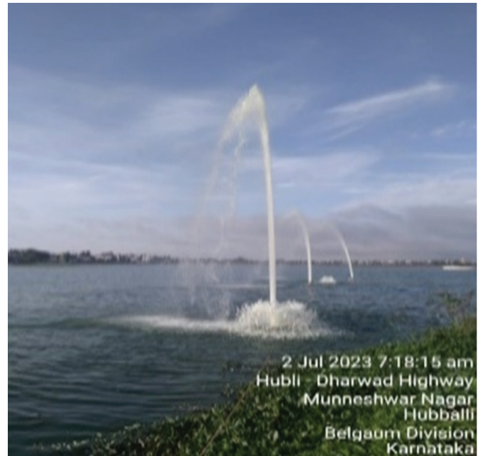
Photograph-2: Diffused Aerators
