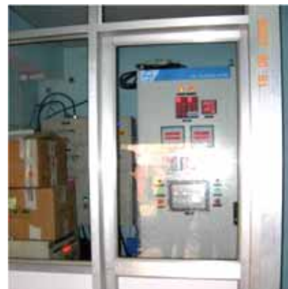
RTU at Distribution Tank
