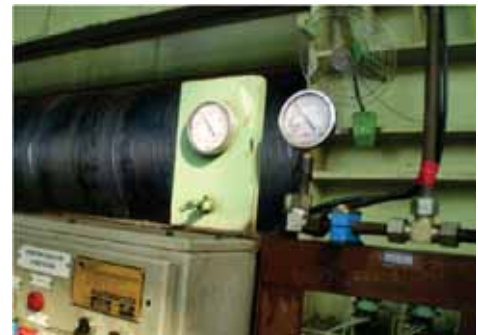
Water Asset Management showing Pressure Gauges
