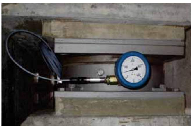
Figure 4. The ongoing condition of the Pont Nanin structure in the Swiss Alps has been monitored by an SHM system (with force monitoring at bearings as shown) since its static design was changed a decade ago (fixing at end).
