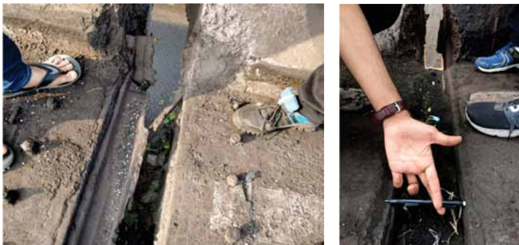
Fig. 2 & 3: Condition of Expansion Joint
