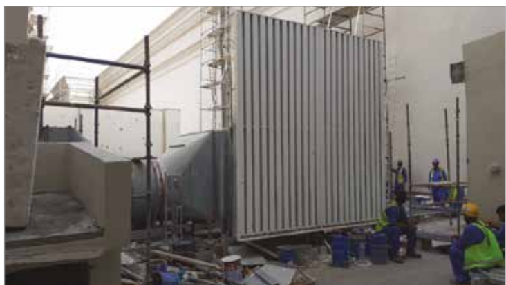
Photo 03: Hazardous Wastes in a construction area
