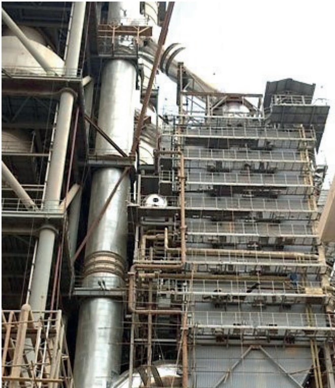
Pre heater Boiler
