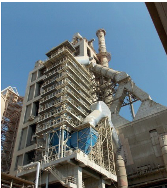
Alkali/ Chlorides Bypass Boiler
