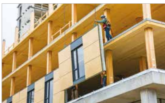
CLT Wall Panels erection [5] CLT panel for Brock Commons in Vancouver (Courtesy: Naturally Wood).
