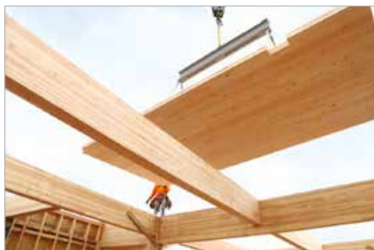
Beam and Slab Panels [4] Courtesy: Contractors install CLT at the LEVER Architecture-designed Albina Yard in Portland, Oregon. (LEVER Architecture)
