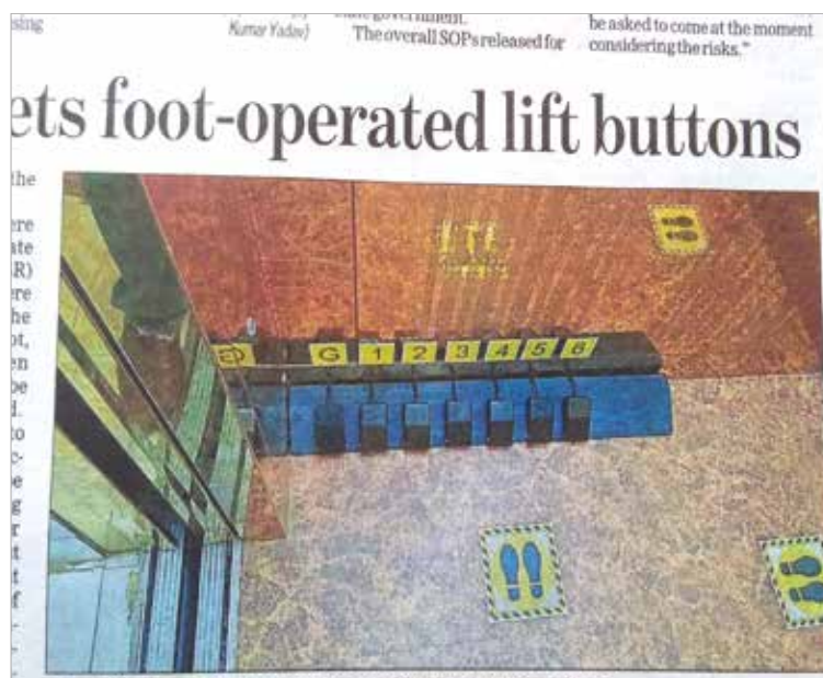
Figure 4: Picture showing pedal operator being installed inside an Elevator/ Lift car (source: local newspaper)
