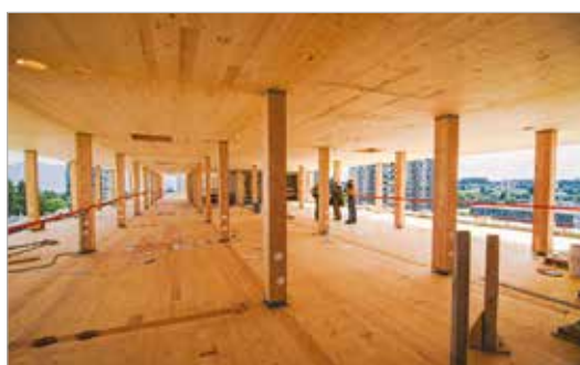
Column and Slab construction [6] Courtesy: Construction on Brock Commons, an 18-storey mass timber building at the University of British Columbia. (SUPPLIED / Postmedia
