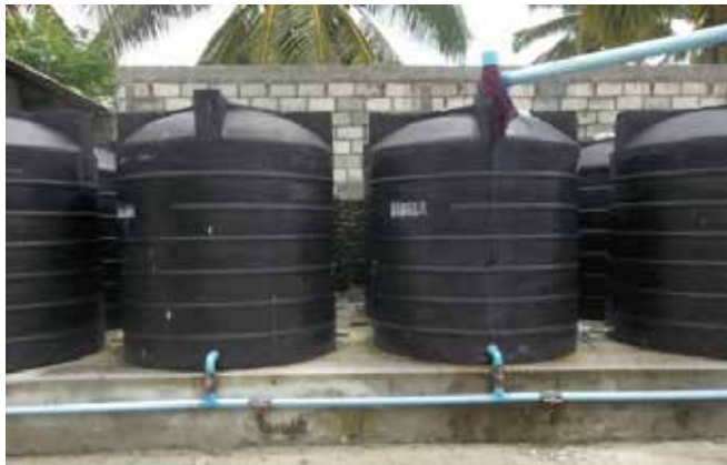
Existing Rainwater Storage Tanks
