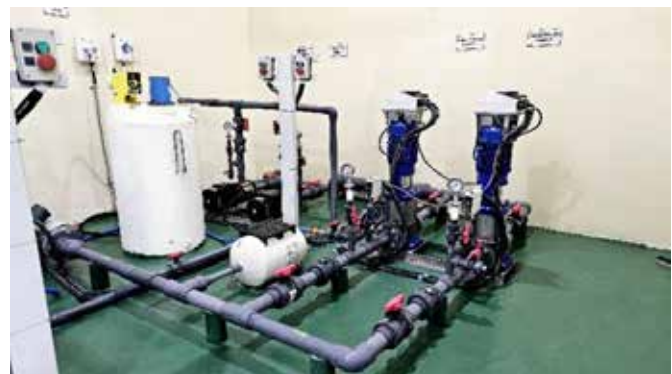
Pumping System for Distribution
