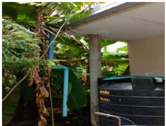
Existing Roof Top Harvesting System
