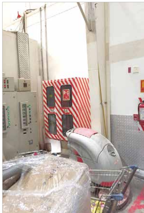
Area & Approach to Fire Hydrant Obstructed (can't be accessed when needed)
