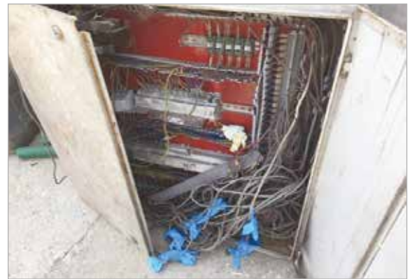
Unkempt Electrical Panel
