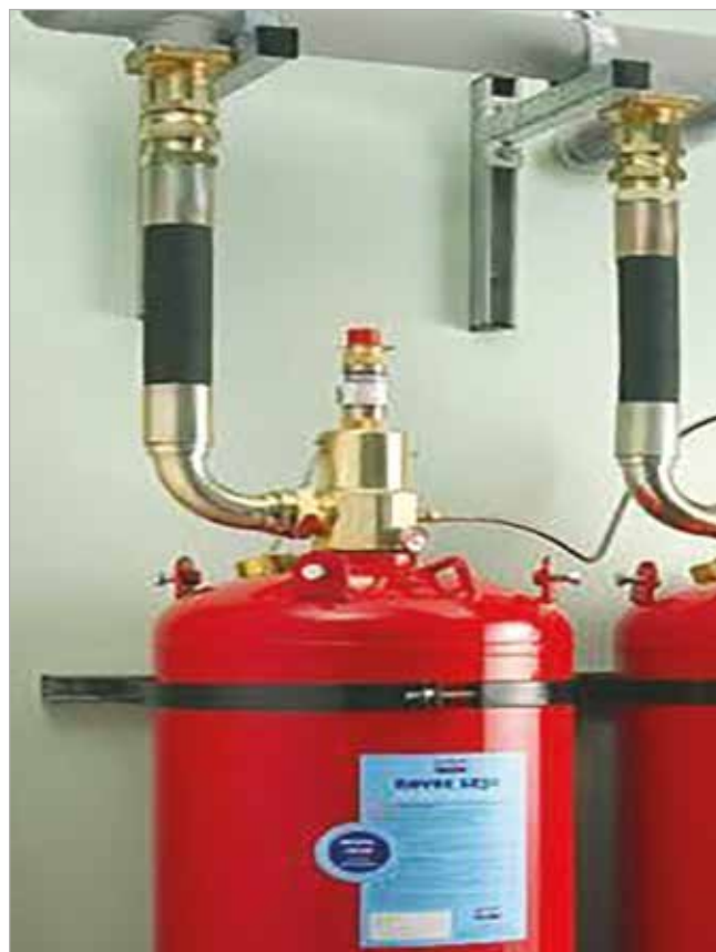
Gas Suppression System - Audible (discharge siren) and visual alarm
