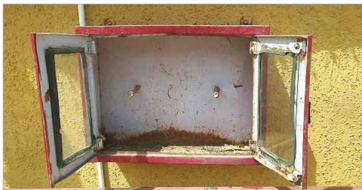
(a) Empty Hose Box - No Hose & Nozzle.
