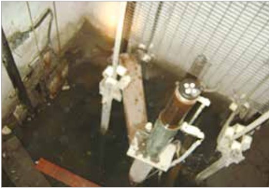
Water in the hoistway pit
