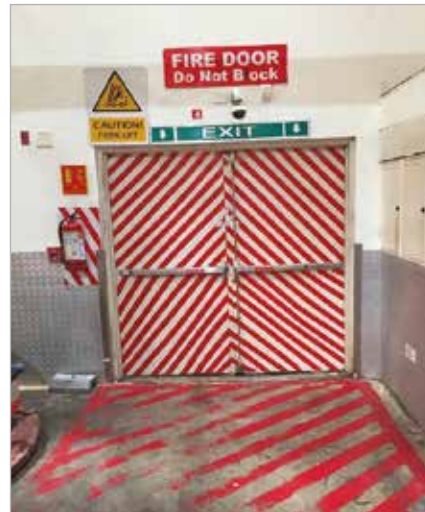
Exit Signage marked in a premises
