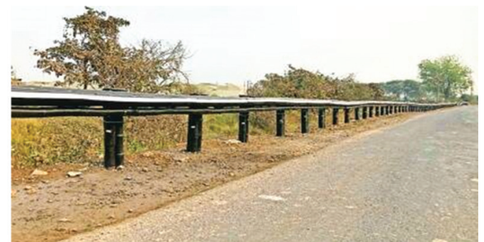
Figure- 5: Bamboo Crash Barrier in Indian Highways (used 1st time in the World)
