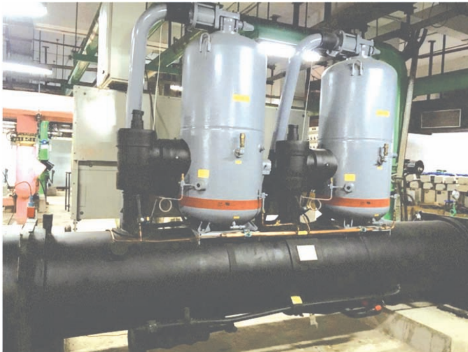
Photograph: 265 TR Non-VFD Chiller
