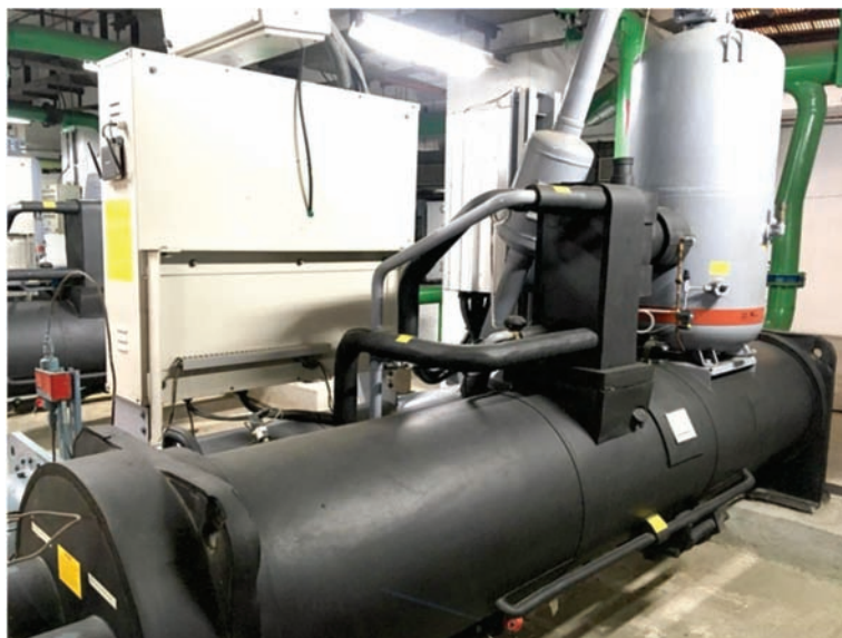
Photograph: 240 TR VFD Chiller
