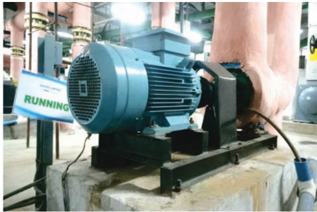
Photograph: Primary Chilled Water Pump
