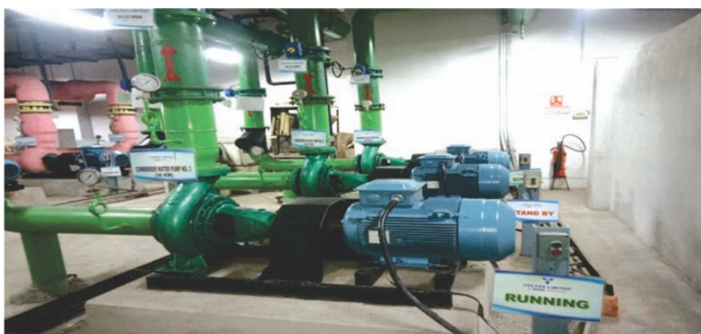
Photograph: Condenser Pumps
