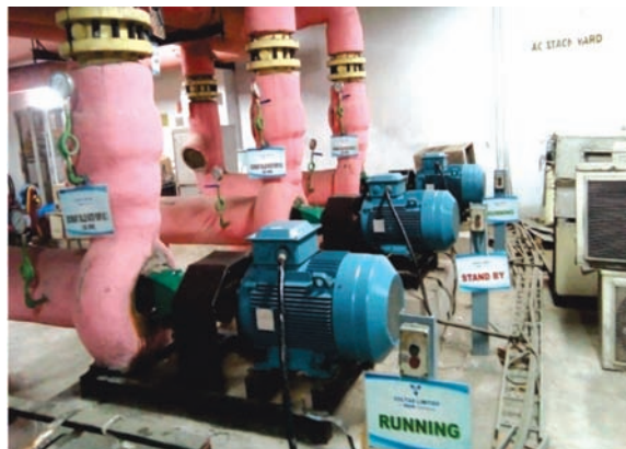
Photograph: Secondary Chilled Water Pump
