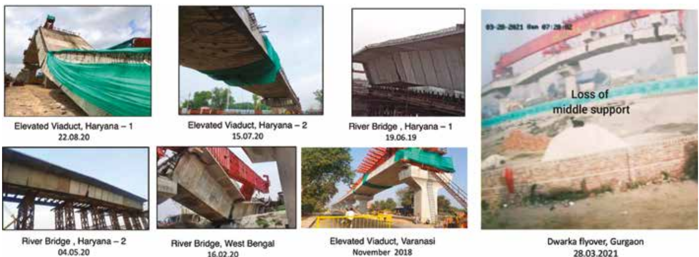
Figure-1: Precast Segmental superstructure failures during construction
